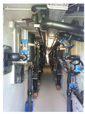
Figure 1: The distribution system for loading and O&M of the DWWT-technologies at the BDZ.
